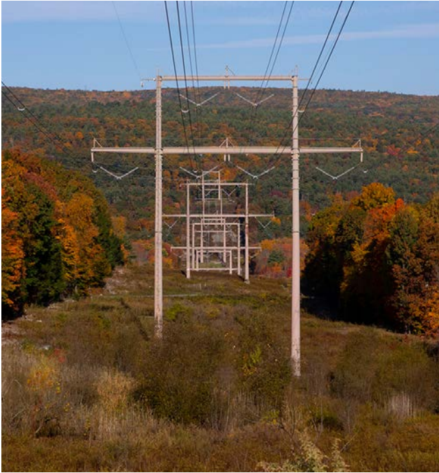
View of CCRT 21/04 of the NYPA-owned 345 KV transmission system at Route 209 near Otisville, looking west. Photo by Philip Kamrass/ New York Power Authority.
