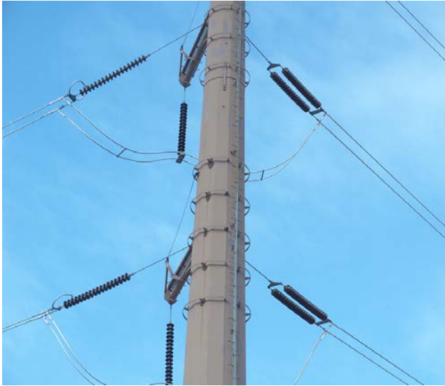
Utilities must place a high importance on knowing the condition of transmission conductors, which are always susceptible to axial, bending moment and shear stresses as well as causing or experiencing cascading power failures. Photo by NYPA.
