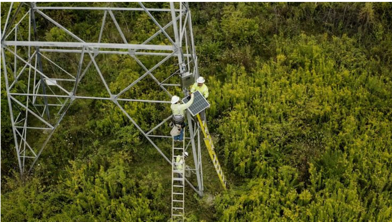
2. Workers install dynamic line rating sensors on an AES Indiana line. Courtesy: AES/LineVision
